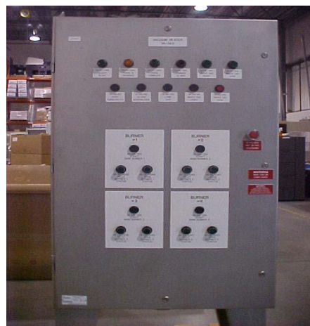
PLC Panel with Push Buttons
